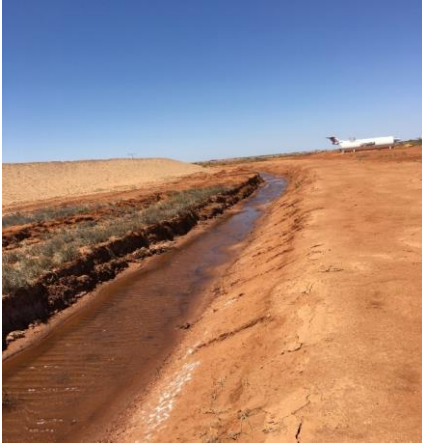
Drain installed in Onslow near airport to drain swamp created by deposited dredging material
